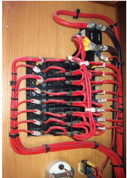
Tidy, correct installation of wiring is important. Photo: Narrowboat Surveys
